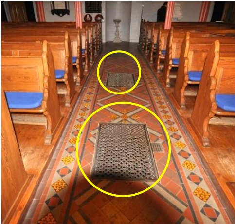
Figure 3. Inlet and outlet grills for the hot air heating system in Enniskillen cathedral
