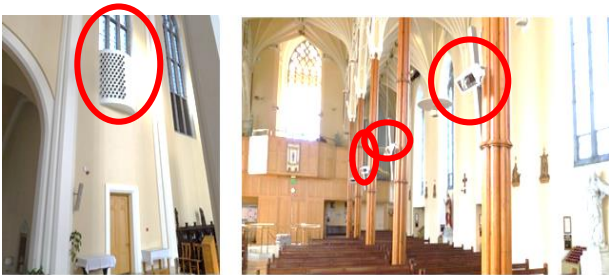
Figure 4. Hot air blower outlet (left) and electric radiant heaters (right) in St. Mary's Cathedral, Cork
