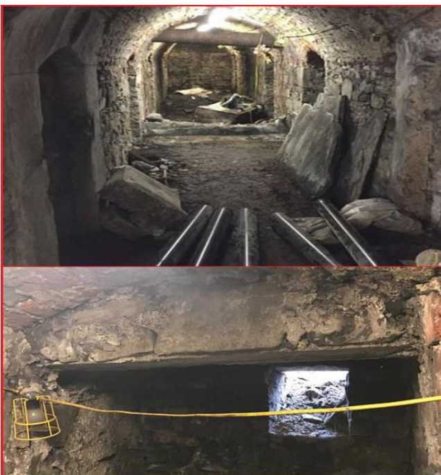
Figure 10: Circulation space within the barrel-vaulted crypt passage (top), and existing ope used for routing of services (bottom) – photos provided by CORA Consulting Engineers.
