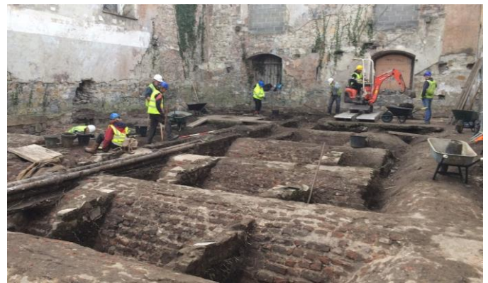
Figure 7: Exposed brick vaults on St Luke's Church project – photo provided by CORA Consulting Engineers.
