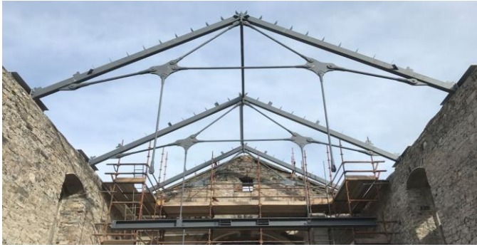
Figure 9: Steel floor beams hanging from the steel truss roof structure – photo provided by CORA Consulting Engineers.
