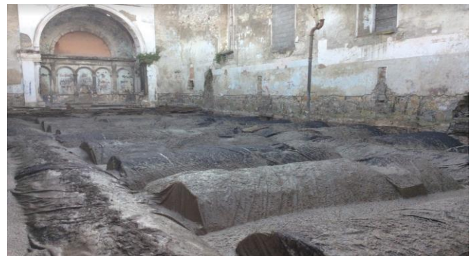
Figure 8: Proprietary fabric membrane dressed over vaults prior to pouring subfloor – photo provided by CORA Consulting Engineers.
