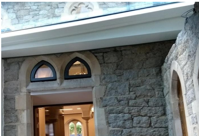
Figure 4: Interface between new façade and existing church at glazed link joining new and old structures – photo by author.
