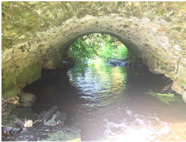
Figure 3. Ballybrogan Bridge before rehabilitation works for severe scour and other defects were undertaken
