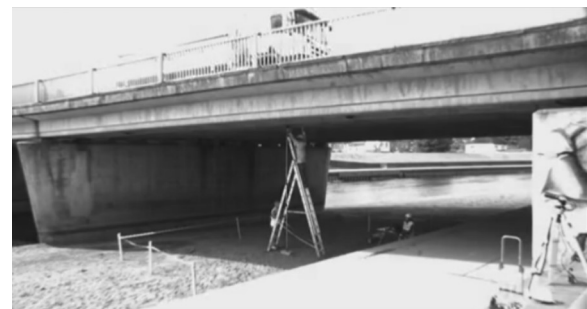
Figure 4. Monitoring installation on bridge as truck passes over midspan during Loaded Swipe 1
